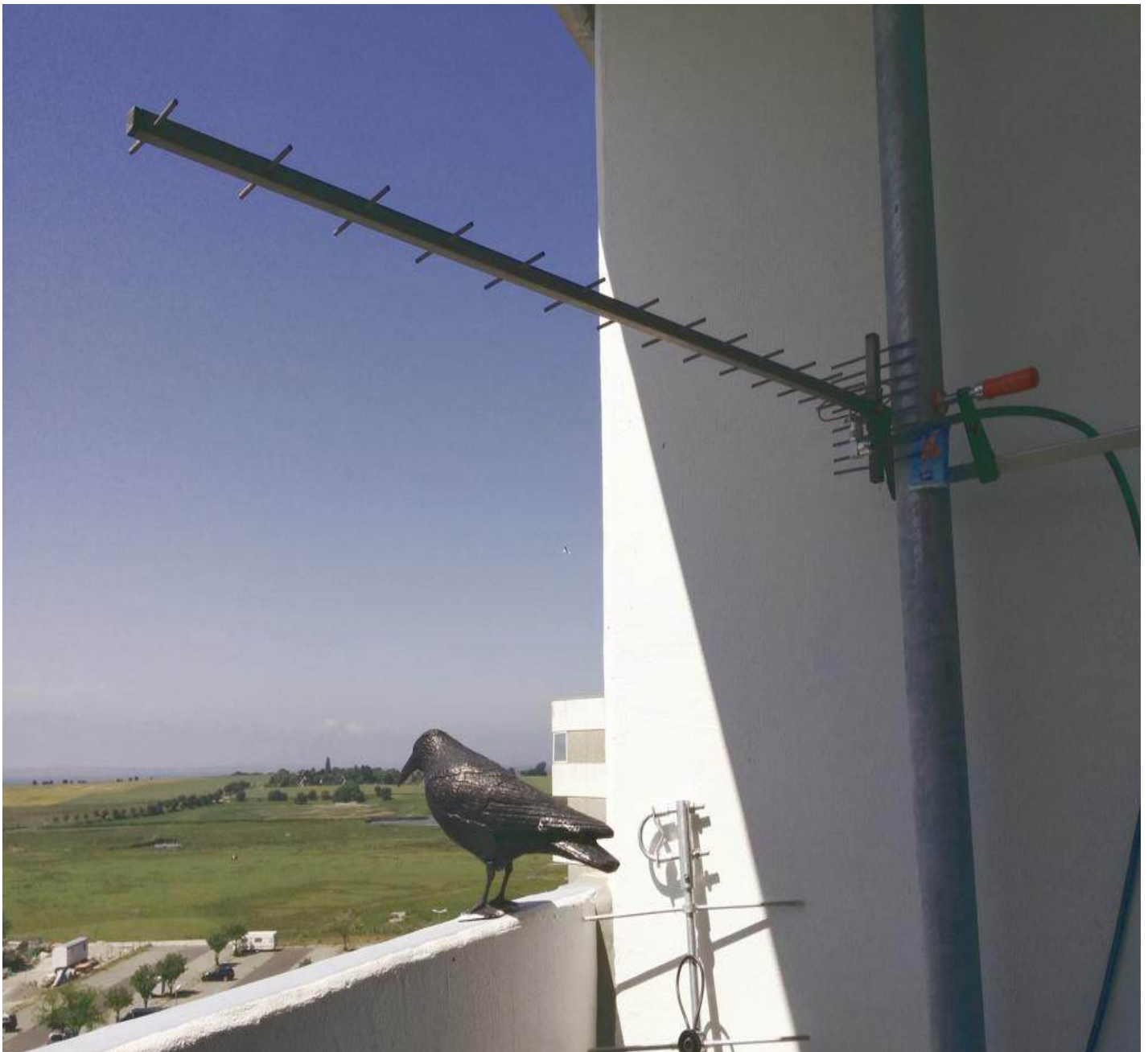
Antenna mounted to rainfall pipe. Baltic sea in the background.
